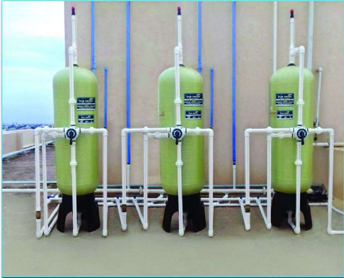
IRON REMOVAL PLANT 5000 L.P.H
