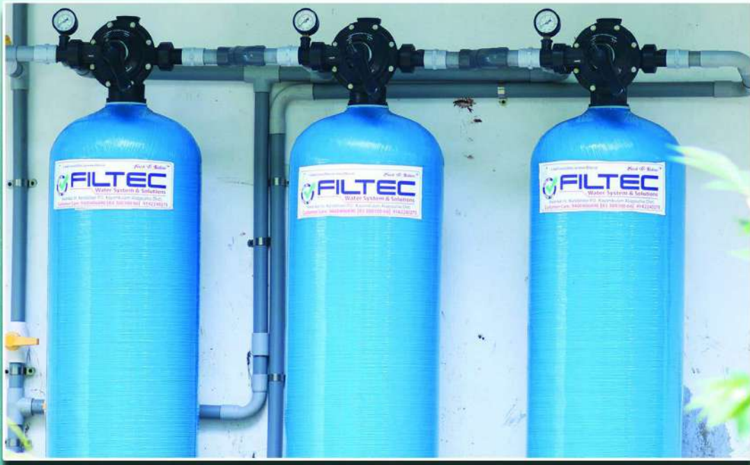
W.T.P. 2500 lph Iron removal plant
