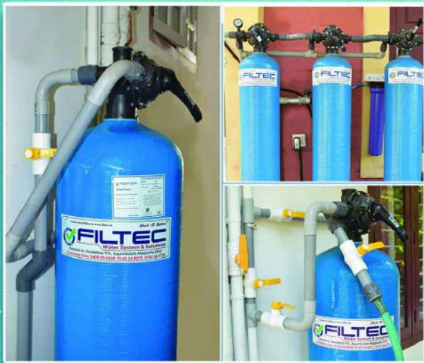
W.T.P. 1000 lph iron removal
