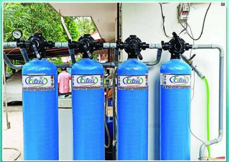
W.T.P. 1500 lph Softner plant
